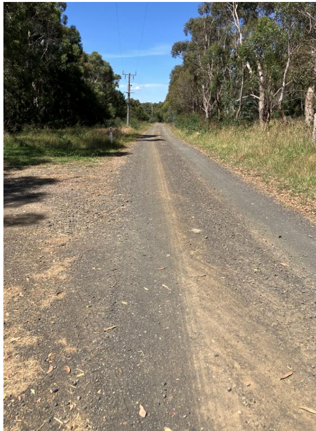
Figure 4 – The existing surface condition of unmaintained Service Lane
