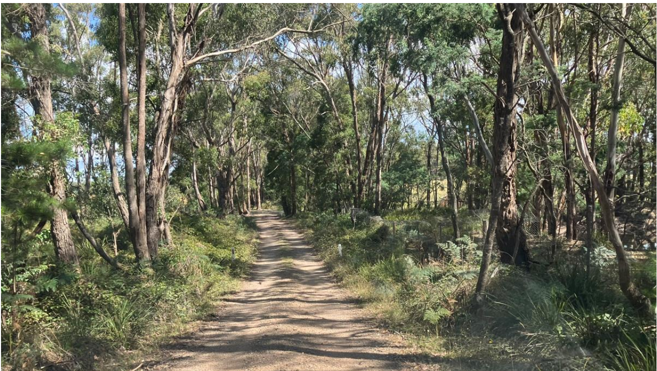
Figure 8 – Poorly maintained existing table drain
