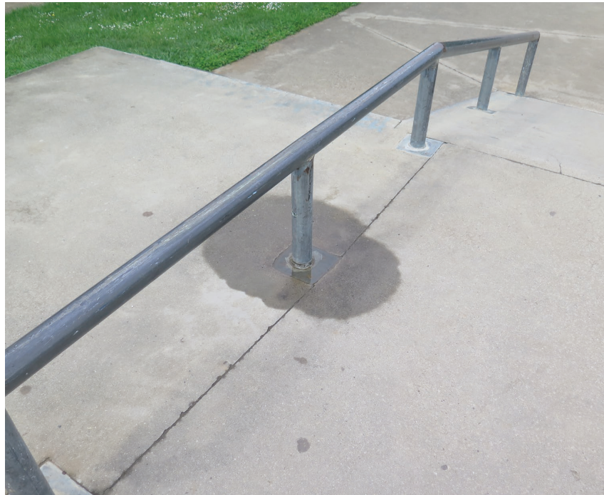
ISSUE: Areas of water ponding SOLUTION: New areas of skatepark to be graded to ensure free drainage. Ensure all existing drainage infrastructure is operational.
