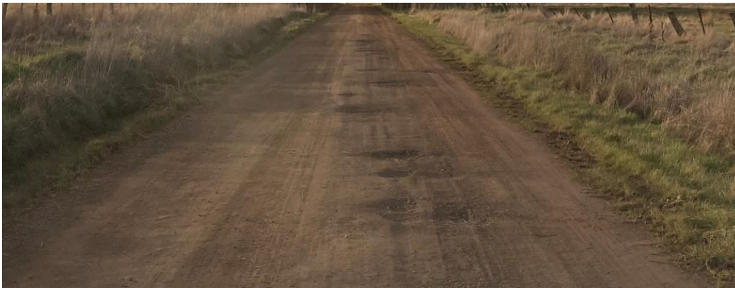
Figure 6 – Typical Potholes 2 of 2
