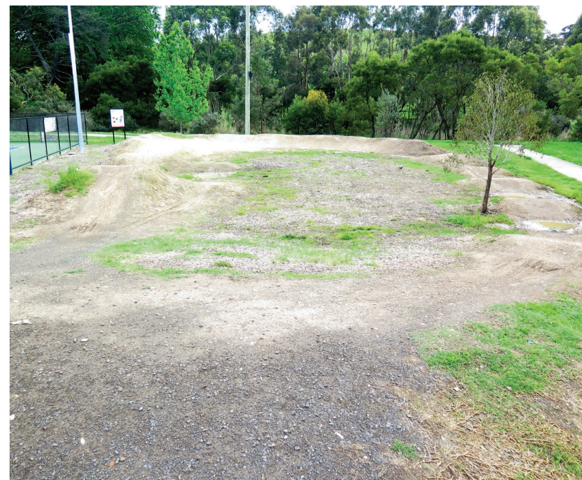
ISSUE: Ponding at bottom of jumps SOLUTION: Include free drainage and where required drainage infrastructure
