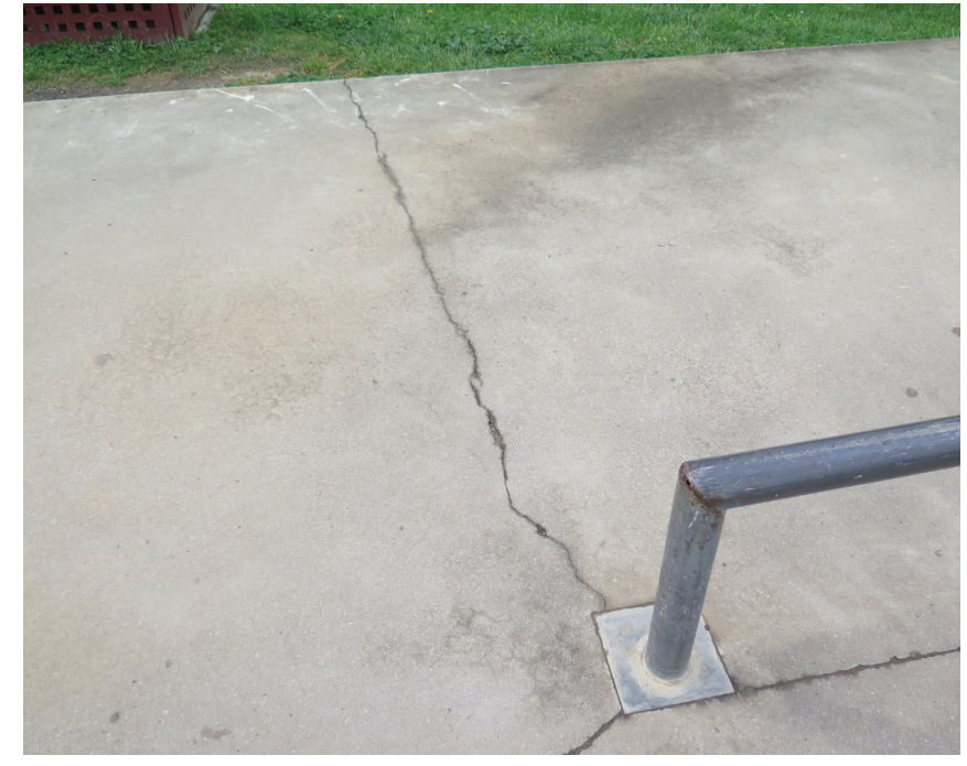
ISSUE: Cracking of concrete on slab SOLUTION: Review all cracks to ensure no vertical displacement. Wide gaps to be filled with epoxy.
