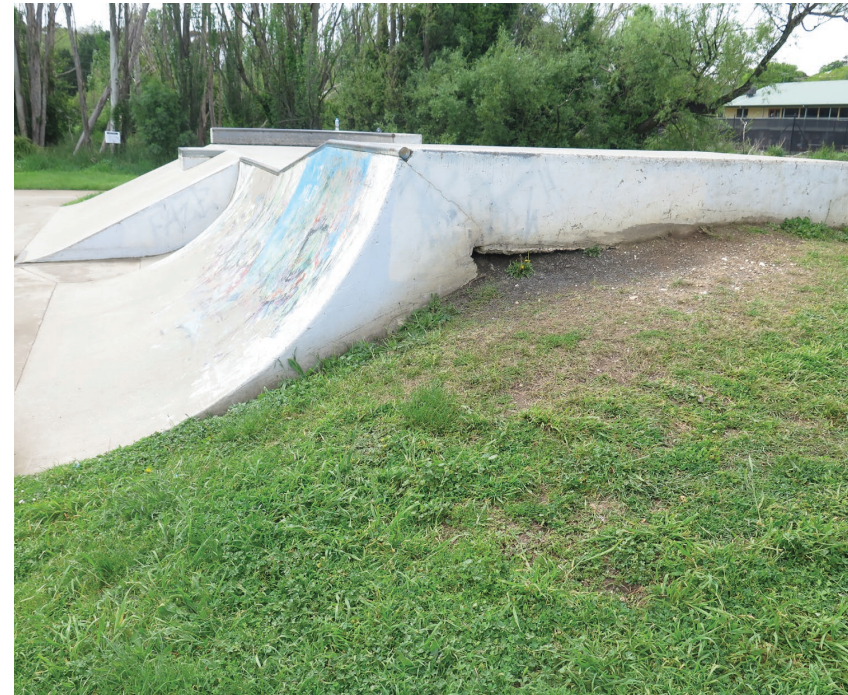
ISSUE: Erosion causing exposure to underside of slab SOLUTION: Upgrade all batters to ensure stability and leveling
