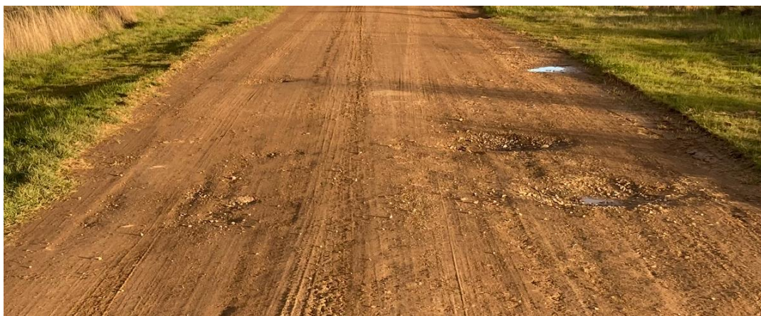
Figure 5 – Typical Potholes 1 of 2
