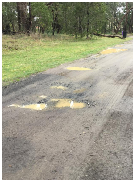
Image 6 – Series of Potholes
