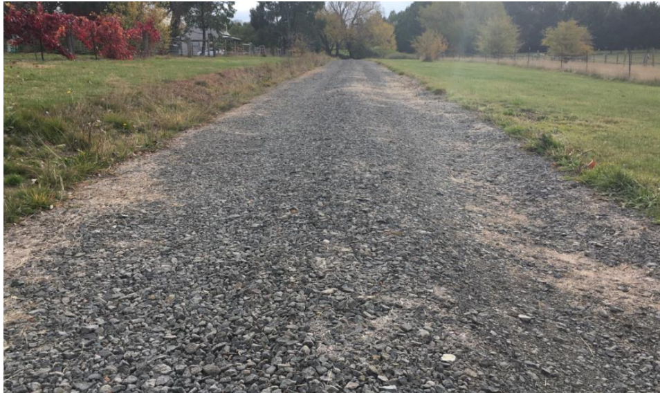
Image 3 – Subject Road, Rutting and Roads Shape Loss
