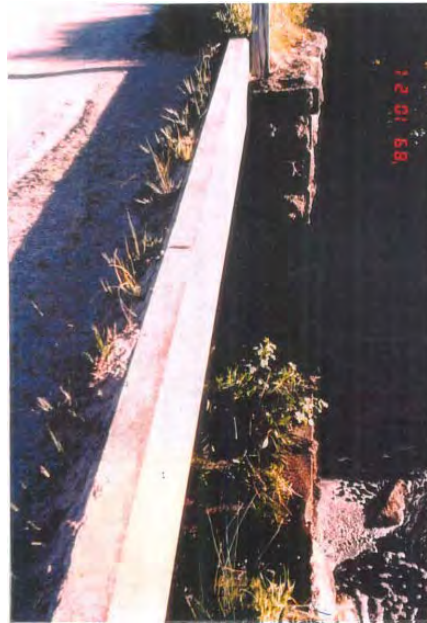
Figures 11 & 12. (L) Stone Bridge Abutments and Piers, Hodges Bridge, Boundary Road, Edgecombe (HO20), Note: 20th century timber deck and balustrade (R) Bluestone Road Bridge Abutments, Central Road, Kyneton South (HO47) (Source: D Bick et al, Kyneton Conservation Heritage Study , vol 6, 1990)
