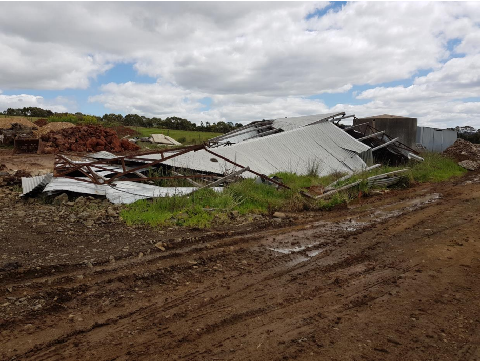
Storm damaged shed.
