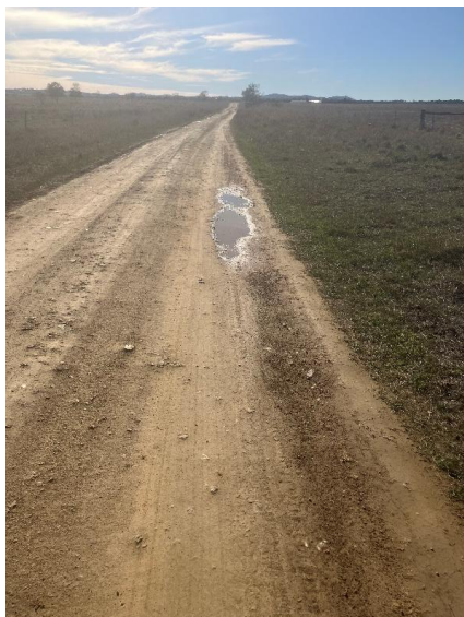
Photo 2: Surface water tracking/ponding along the wheel track
