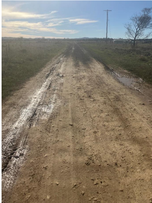
Photo 3: Surface water tracking/ponding along the wheel track due to a lack of swale drains and adequate surface flow management
