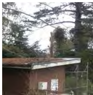
Image 26. Pump House and tank within security fencing
