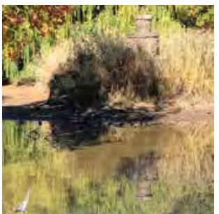
Image 9. Fountain requires repair, possible habitat opportunities on island
