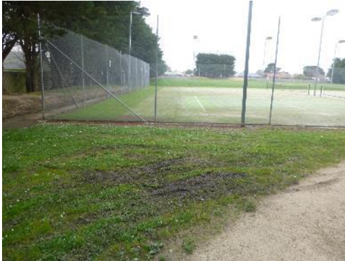
Drainage issue near the courts
