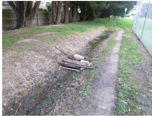
An open drain
