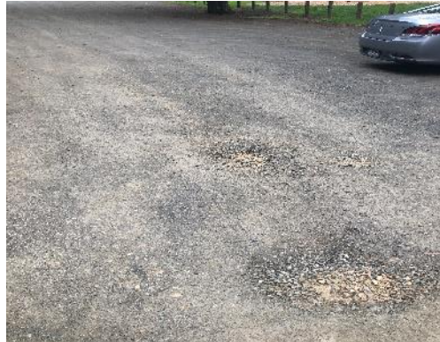
Some potholes in carpark but not too
