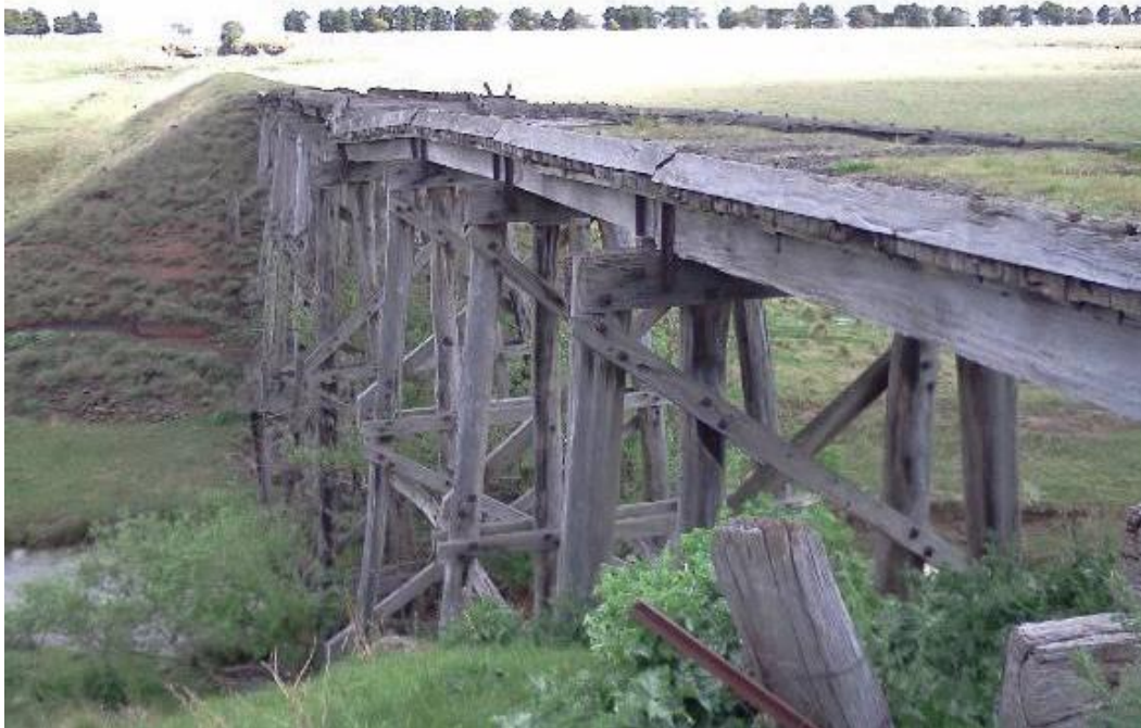
Figure 3.8 Bolinda Creek Viaduct, built in the early 1880s. (National Trust of Australia (Vic) Register, B3033)
