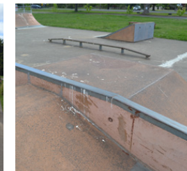
Cracking / rough surfacing on obstacles.
