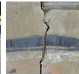
Concrete cracking at joints.
