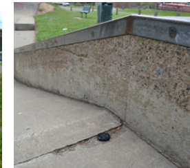
Cracking / surface damage at joints.
