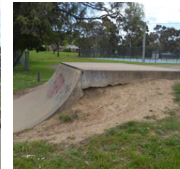
Erosion of earthworks around skatepark.
