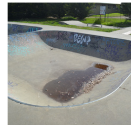
Pooling of water at base of bowl.
