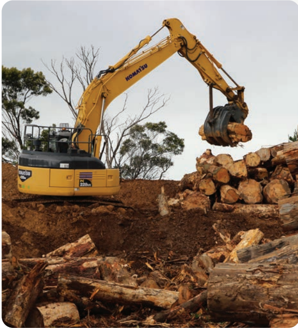
Storm recovery, Romsey
