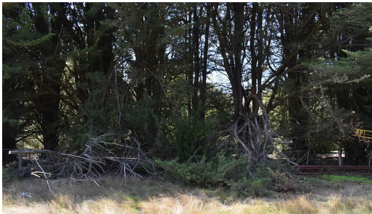
Figure 5 Cypress windrow along the eastern boundary with large failed stems and branches throughout
