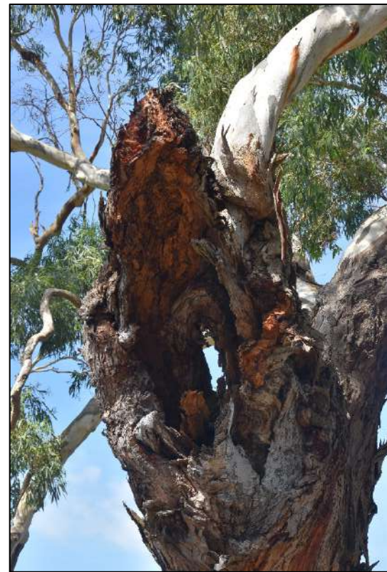
Showing the attachment of the second branch with extensive decay throughout the previously failed trunk.
