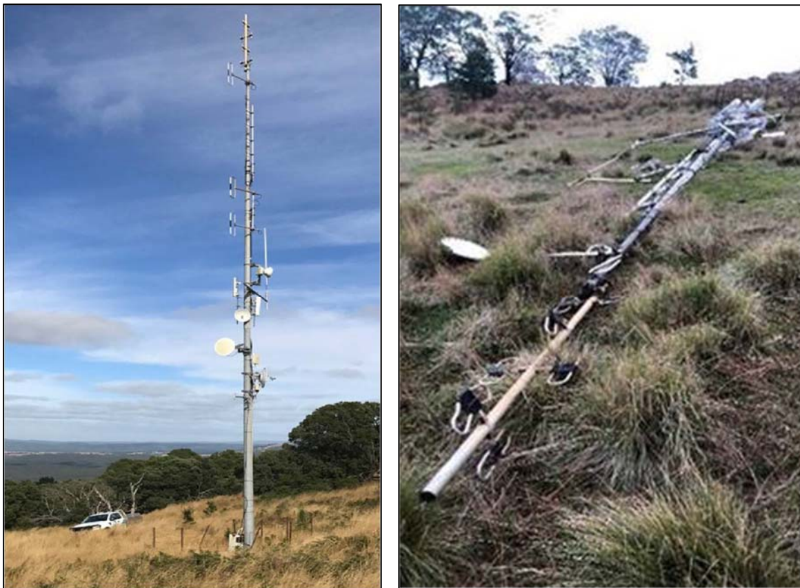
Figure 4: Mount Gisborne tower before and after structural failure
