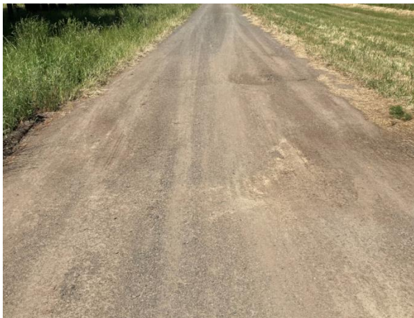
Figure 5 – Road in a state of disrepair
