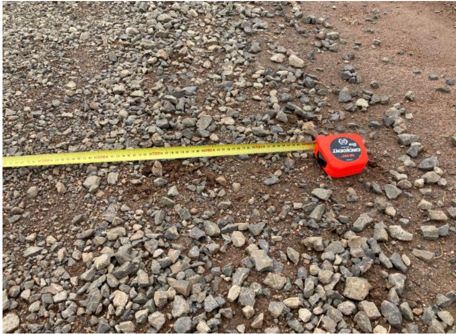
Figure 6 – Road Base exposed under a thin layer of crushed rock
