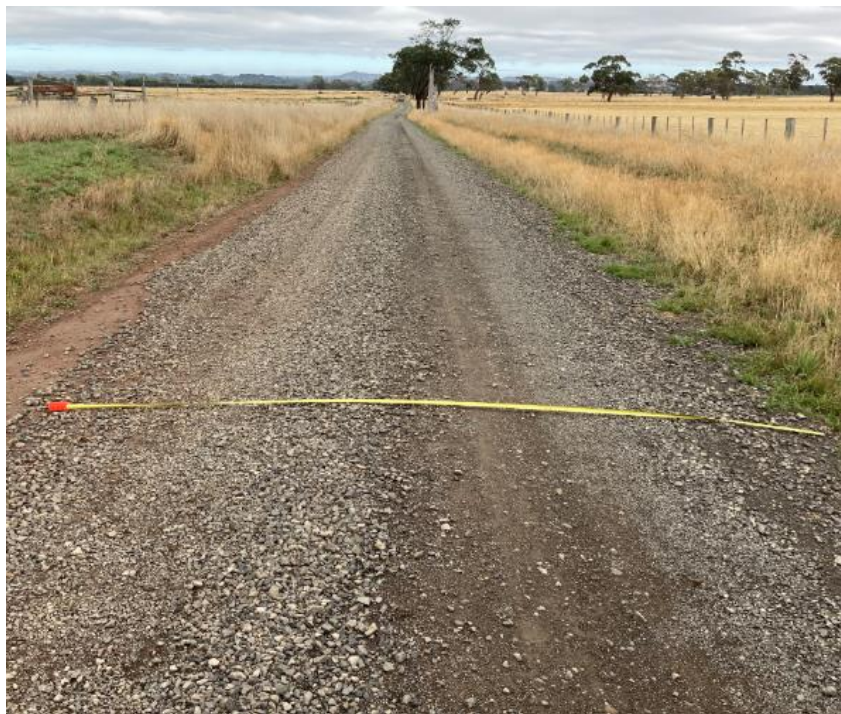
Figure 7 – Gravel loss and minor deformation of pavement
