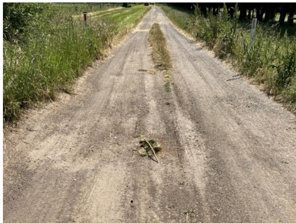
Figure 6 – Road in a state of disrepair
